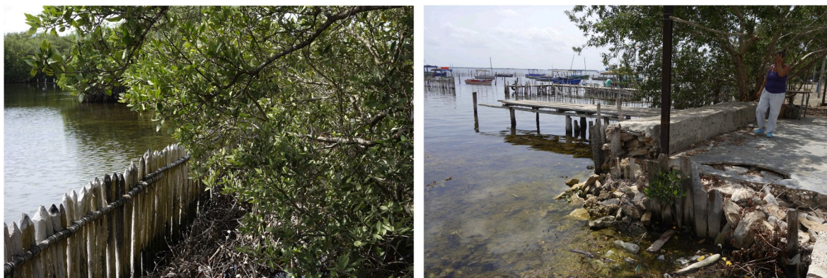
Fig. 3. Barriers built by residents to prevent flooding. Left: made of wood. Right: stone.
