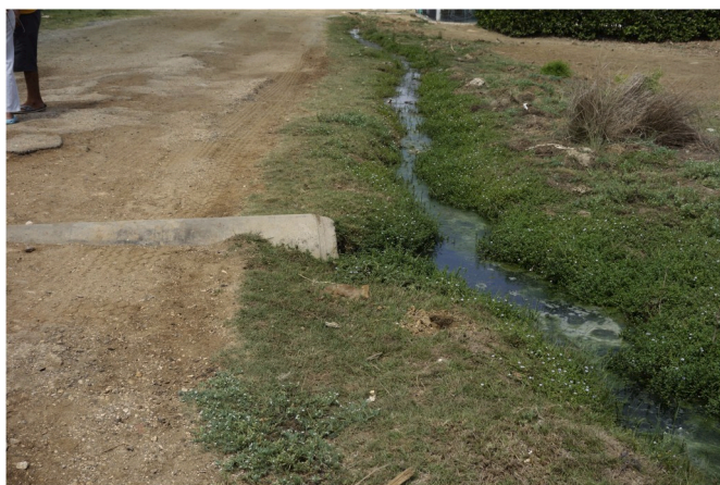
Fig. 4. Ditch and canals built by residents to prevent flooding on a main road.
